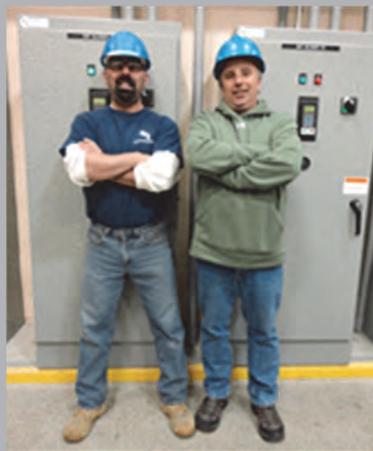
Tom Therrien and Kevin Joerres strike identical poses in front of two of the many panels rebuilt following the flood.
