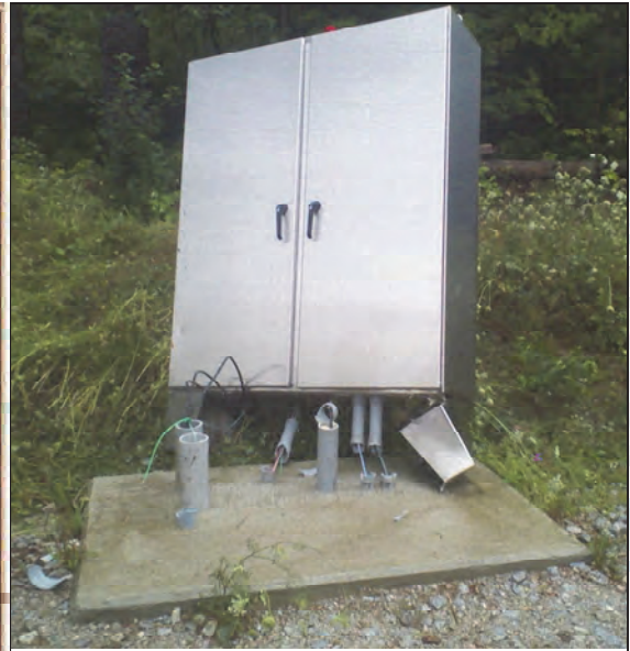
North Conway, NH— Automobile vs. Control Panel ends badly.
