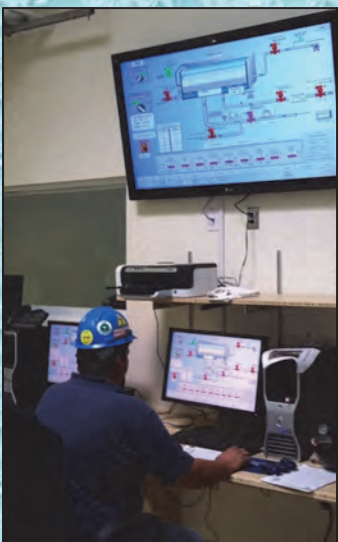
Jim Fritz monitors one of the new plant's first backwash cycles.
